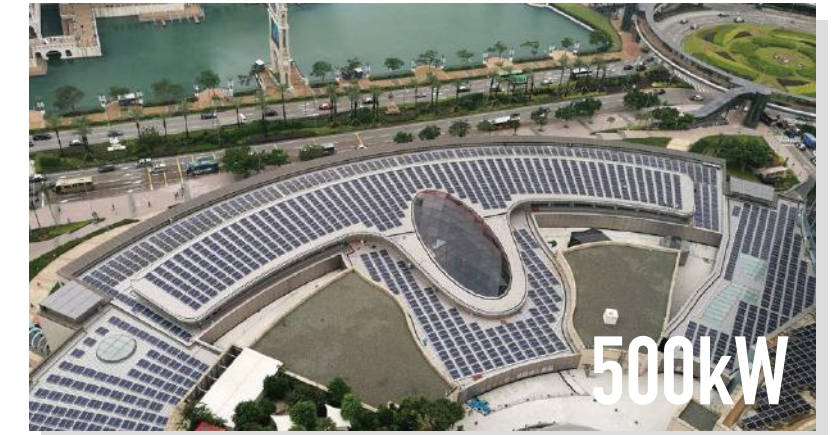
Project Type: Commercial Rooftop Location: China / Macao Commission Date: 2018-4 Product: SRP-300-6MB
