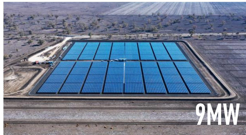
Project Type: G-Mounted Location: Australia / New South Wales Commission Date: 2019-5 Product: SRP-325-6PA MX
