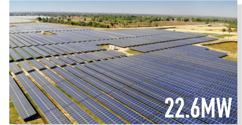
Project Type: G-Mounted Location: Cambodia / Kampong Speu Commission Date: 2020-1 Product: SRP-335-BPA
