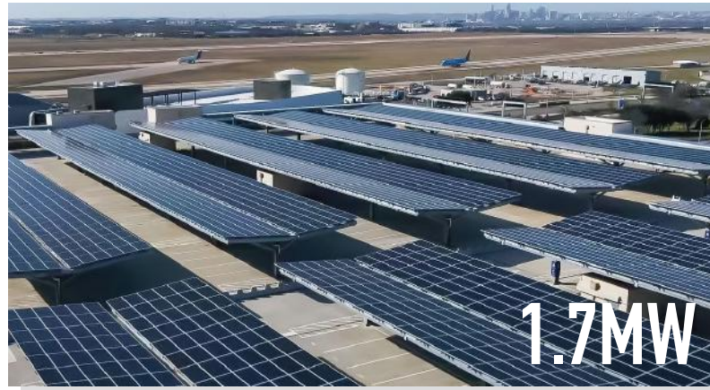
Project Type: Commercial Rooftop Location: USA / Austin Commission Date: 2022-1 Product: SRP-345-6MA
